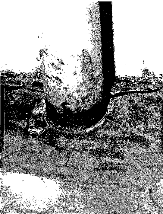
Fig. 3. Cracks and edge rising at the end of flooring.
